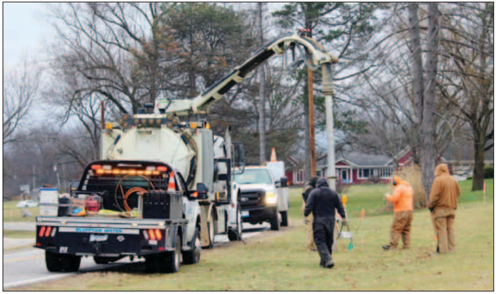
City of Bluffton employees install lighting poles on River Road Thursday morning. (Photo by Holly Gaskill)
