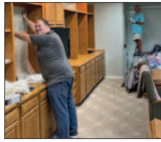
Painting and shelf repair were the projects at Grace & Mercy's reception room. Workers were Dan Lautzenheiser, at left, and George Babcock on the ladder at right.
