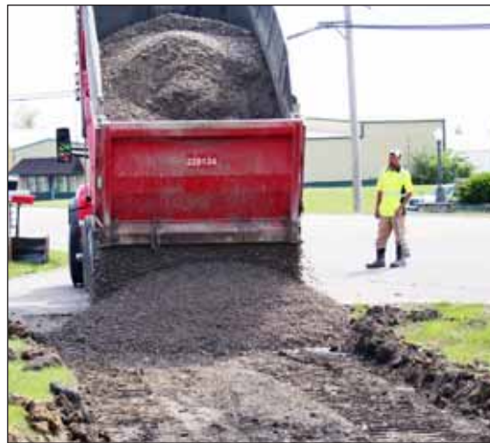
Work on the Interurban Trail Extension began in April as crews began digging and leveling out the trail. (News-Banner file photo)
