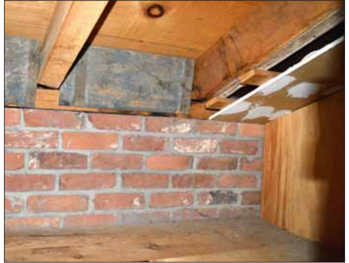
Inside the "garrett," a secret hiding place in the servant's quarters of the Levi Coffin Home in Fountain City, where 14 fugitives once hid to elude slave hunters.
