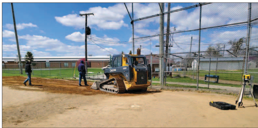
Crews of volunteers work to make needed repairs at the Ossian ball diamonds. (Photo submitted)
