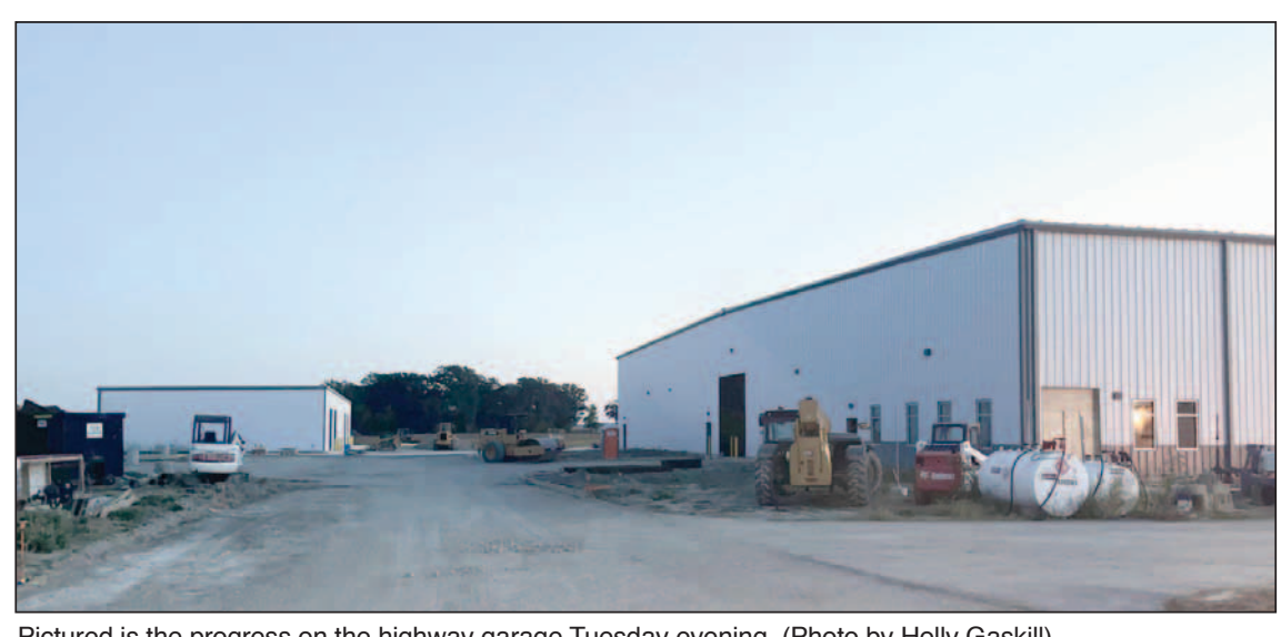
Pictured is the progress on the highway garage Tuesday evening. (Photo by Holly Gaskill)
