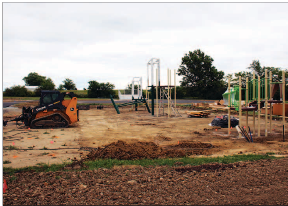
Crews have begun work to install the playground at Lancaster Park, located across from Lancaster Elementary School. (Photo by Holly Gaskill)
