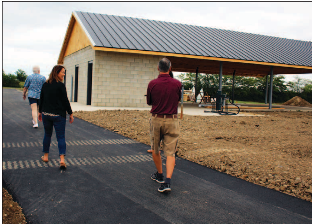
Parks Department Superintendent Brandy Fiechter guided the park board through a tour of the Lancaster Park construction site on Thursday night, highlighting the recent progress made. Pictured, the group takes the walking path to view the pavilion building. (Photo by Holly Gaskill)
