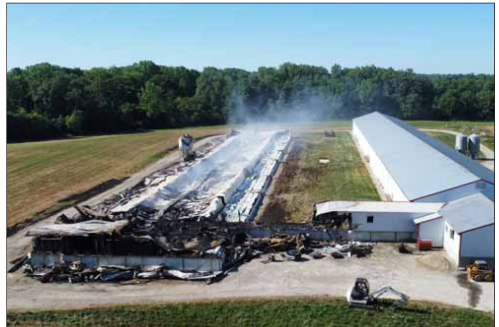
This photo taken by Zane Herr utilizing a drone shows the full extent of the damage to the all-steel building and its close proximity to the “twin” barn to the west. Fortunately, what breeze there was that night was from the west and firefighters focused most of their efforts on keeping the west building covered with water. (Photo provided)
