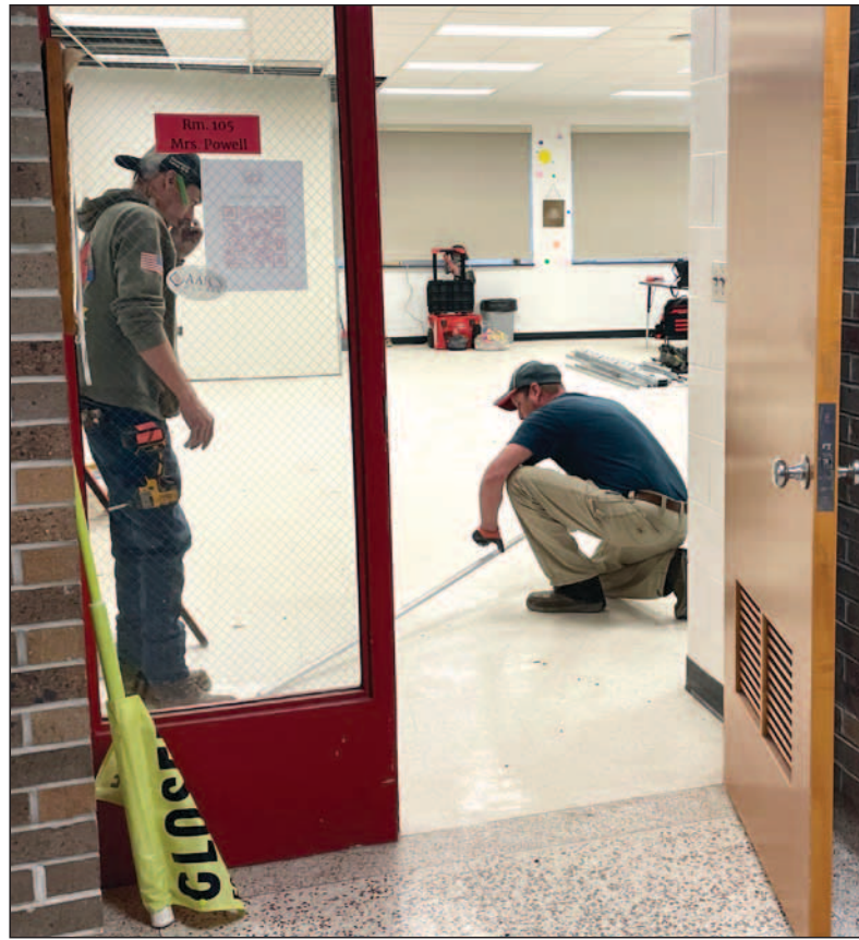
Construction has begun at Southern Wells High School for its new preschool, which will begin next school year. (Photo by Holly Gaskill)
